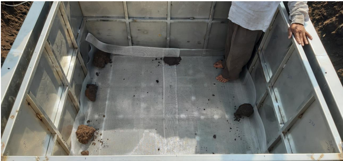
Fig. 10. Placing of mesh at the bottom of inner tank to prevent washing out of soil through drain
