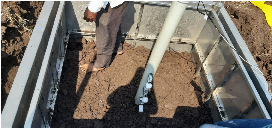
Fig. 11. Layer wise soil refilling & compaction and sensor installation in the inner tank of lysimeter
